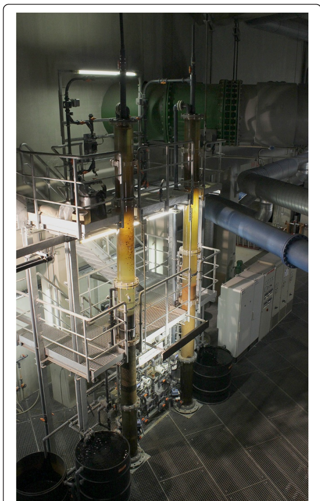
Figure 3 Dual-media rapid filters of the pilot plant in the PEP Tegel in Berlin.
